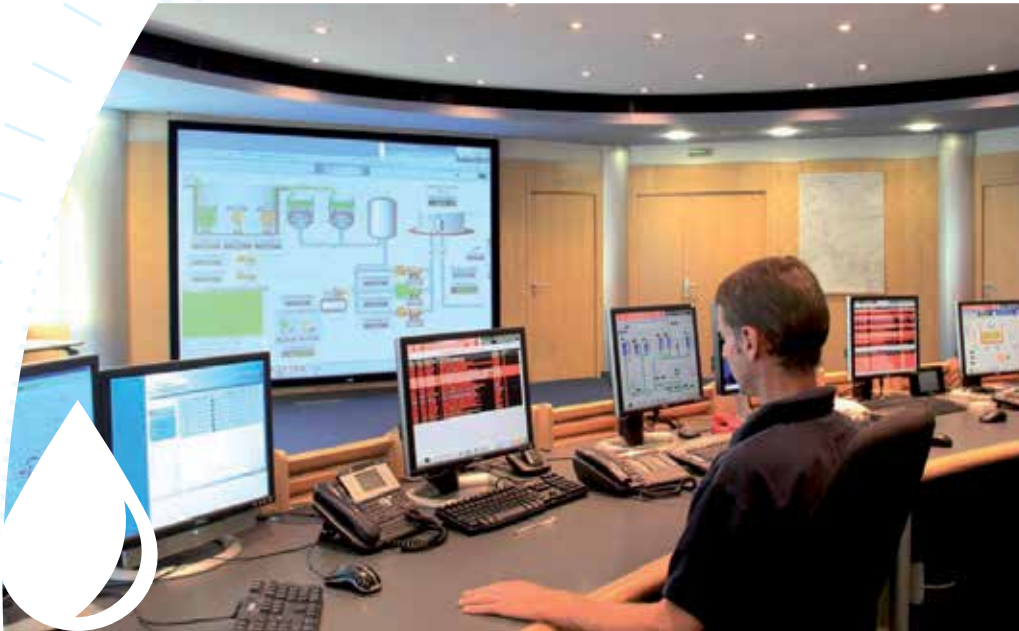
Panorama at the Telemetry Center of the Société des Eaux de Marseille. Permanent remote overseeing of over 850 hydraulic plants, real-time collection and treatment of almost 95,000 data points.
