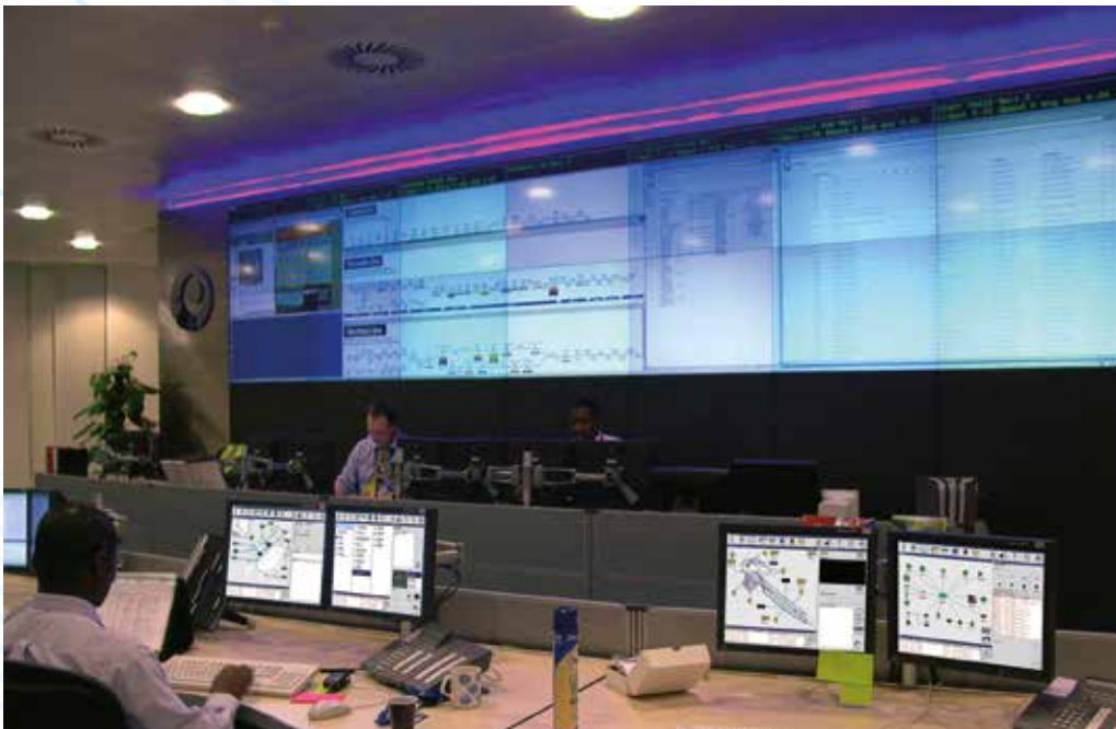
Panorama E 2 used at Tube Lines control center
